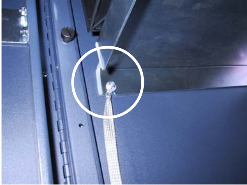
Figure 6. Grounding strap secured to dispenser tray mounting bolt.
