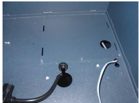
Figure 24. Power supply and dispenser data cable removed from cabinet.
