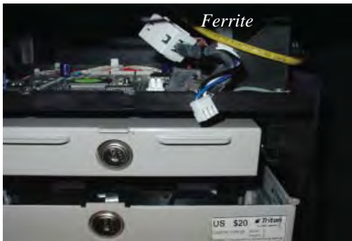
Figure 4. Power and Comm cable disconnected.
