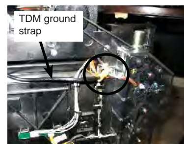
The ground strap connection at the TDM dispenser.
