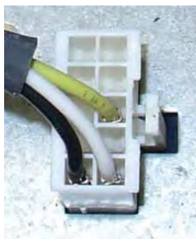
The TDM dispenser DC power cable connection (10-pin connector) at the dual power supply
