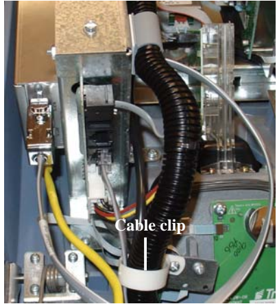
Figure 2-37. External Ethernet cables routed and connected.
