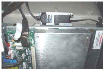
Figure 3. Modem secured and connected.
