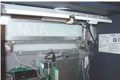
BALLAST/BULB LIGHT PANEL
