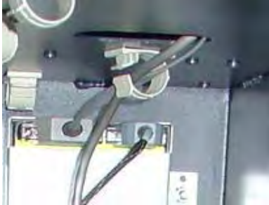
Figure 12. EJ and dispenser power cables.
