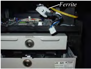
Figure 9. Power and Comm cable disconnected.
