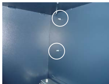
Figure 8. Mounting bolt location.
