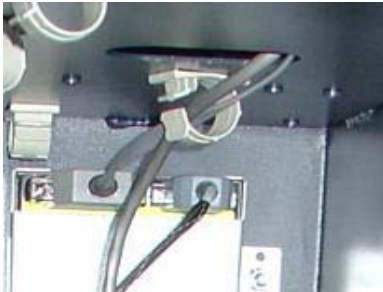
Figure 12. EJ and dispenser power cables.
