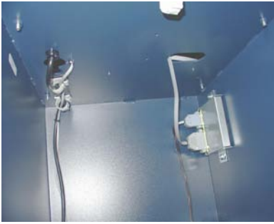
Figure 12. EJ to Docking board cable.
