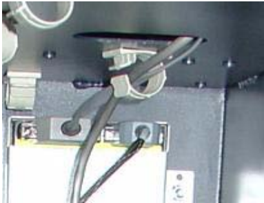
Figure 12. EJ and dispenser power cables.
