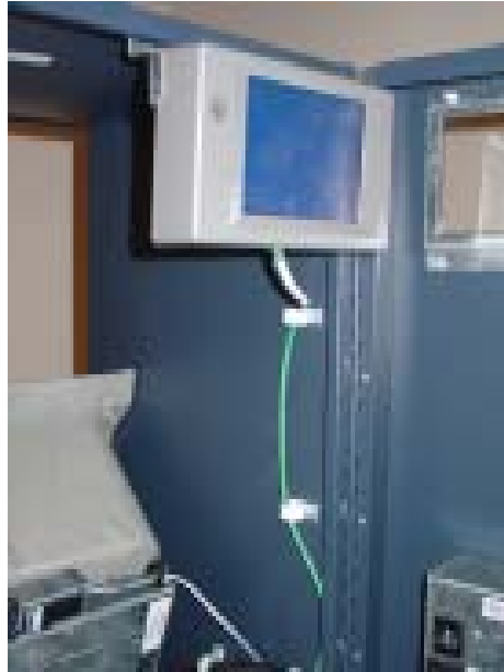
Figure 3. OSP mounted and cable connected.
