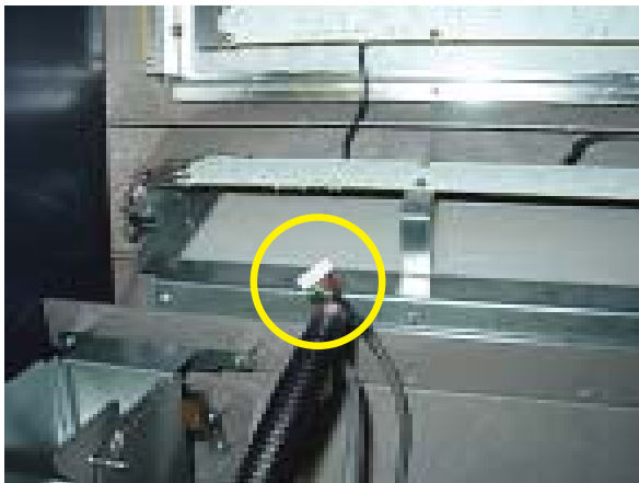
Power cable (located in harness).
