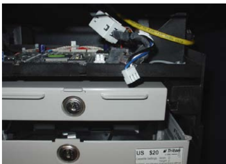
Figure 5. Power and Comm cable disconnected.
